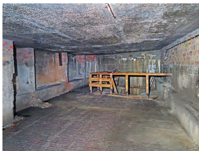
The sump at the lowest level of the Alexanderplatz shelter; the various brick types revealing GDR-era repair and modification. Photo Clive Penfold
